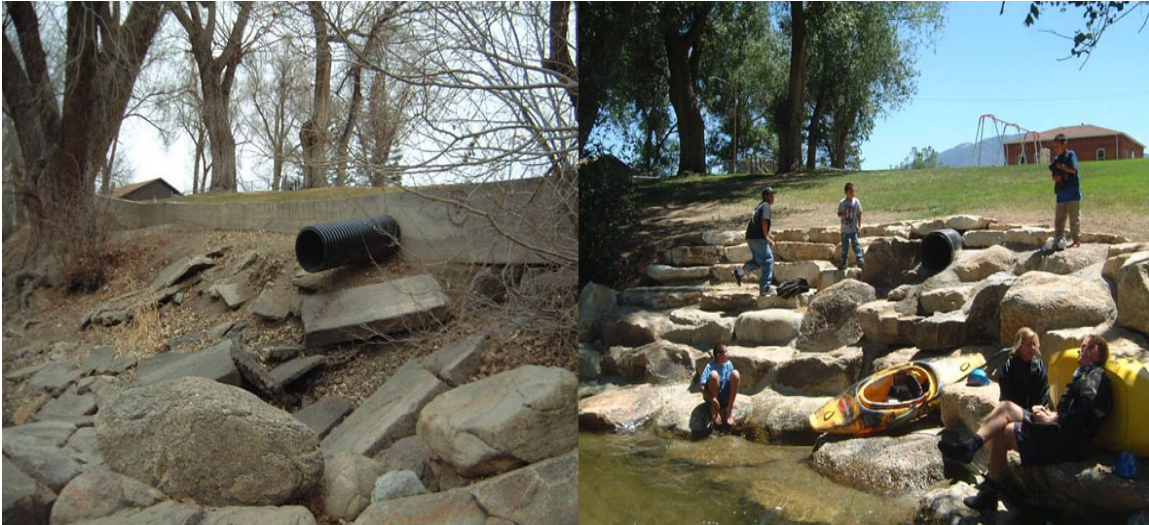
Figure 8. Example of bank terracing replacing an existing wall and stabilizing a stormwater outlet pipe.
